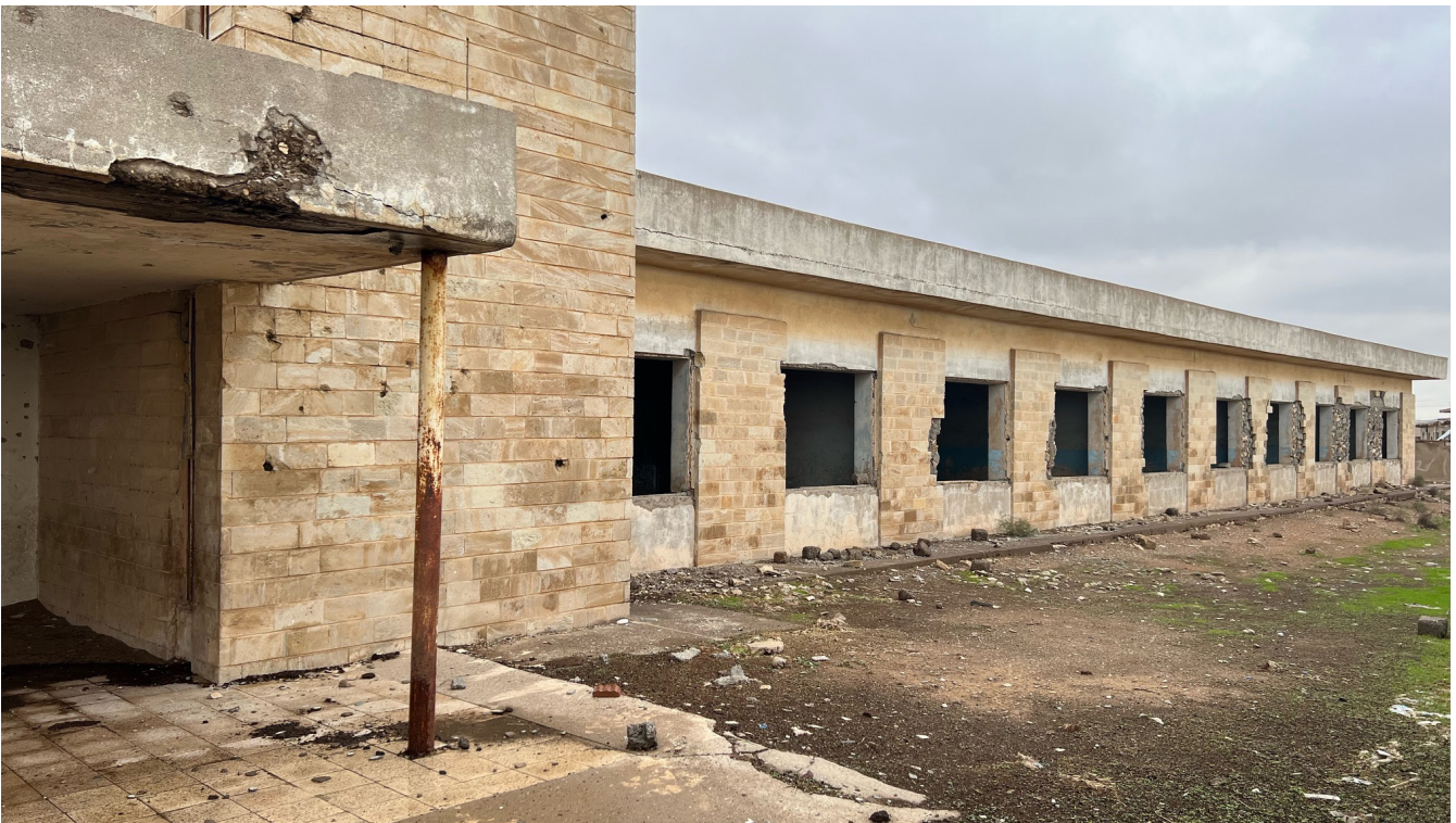
Figure 3: Damaged School in Mangoba
