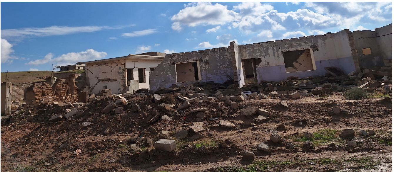
Figure 10: Chamakor Damaged Houses
