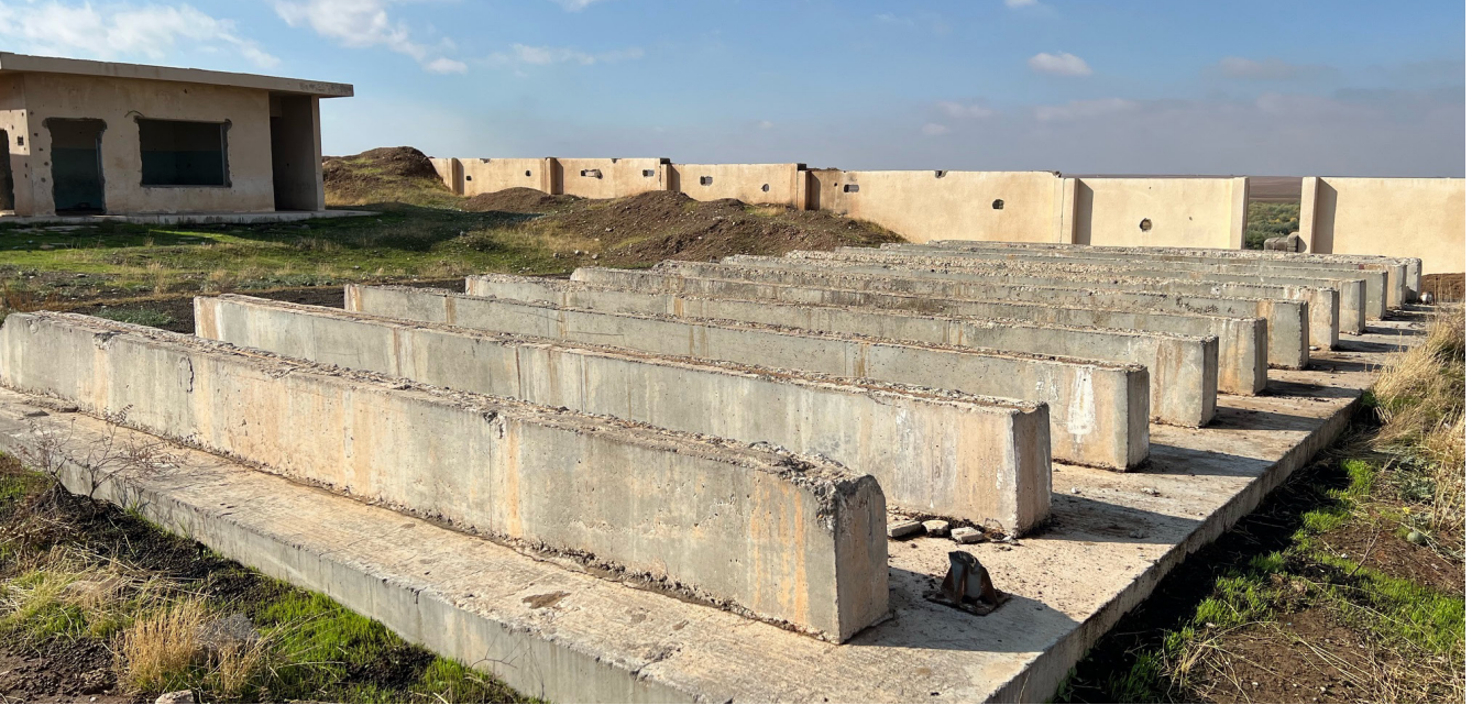
Figure 17: Tal Aswad Saghir Damaged Water Treatment Plant
