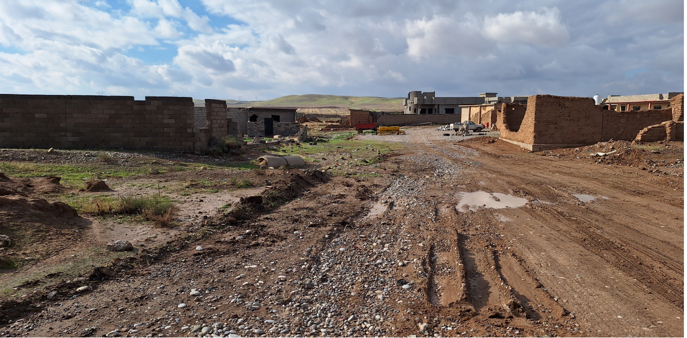
Figure 12: Chamakor Unpaved Internal Road
